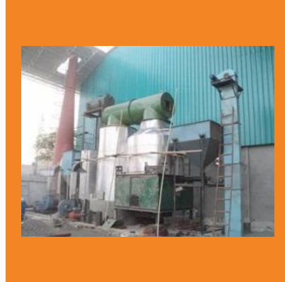
Thermic Fluid Heater
