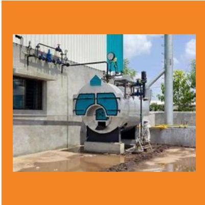
IBR Steam Boiler
