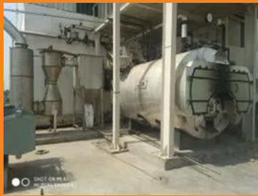
Wood & Coal Fired Steam Boiler
