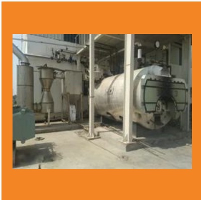
IBR Steam Boiler
